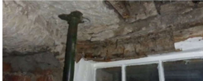
Fig 18. Dry rot cubing to flat entrance lintol
