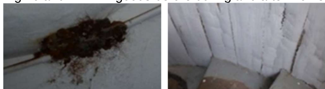
Fig 12 and 13. Dry rot fruiting body, cubed timber in stair
