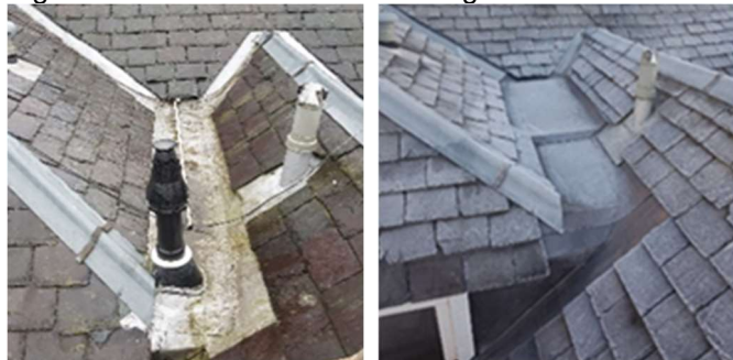
Fig 8 and 9. Gutter detail before and after
