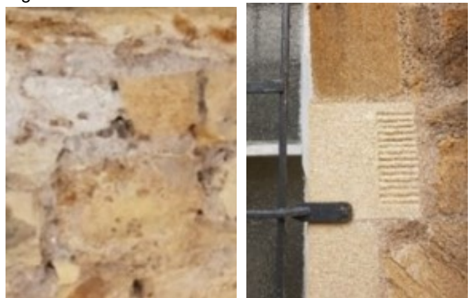
Fig 26 and 27. Evidence of mason bees, grate repair
