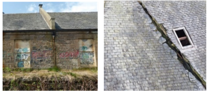
Fig 17 and 18. Graffiti, Warehouse 5 roof collapse
